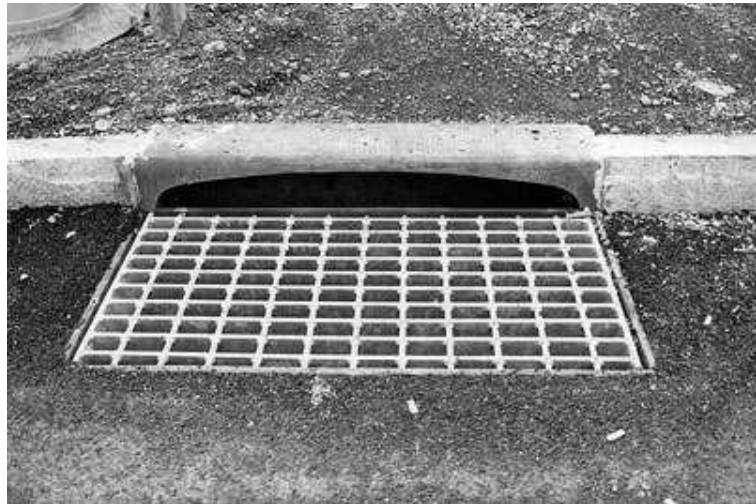
Figure 39: Bicycle Safe Drainage Grates Photo Source: FHWA-SA-09-024
