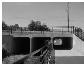
City of Olathe, KS Indian Creek Trail Mur-Len Rd. box culvert underpass Class I Multi Use Path 10 foot.
