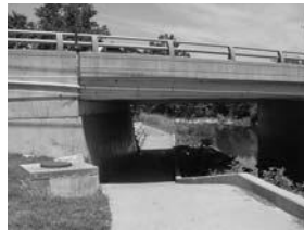
City of Kansas City, MO Indian Creek Trail 103rd St. underpass for concrete Class I Multi Use Path 10 foot.
