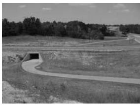
City of Blue Springs, MO Adam’s Dairy Parkway & 1-70 Interchange. Box culvert, Asphalt Path Class I Multi Use Path 10 foot.
