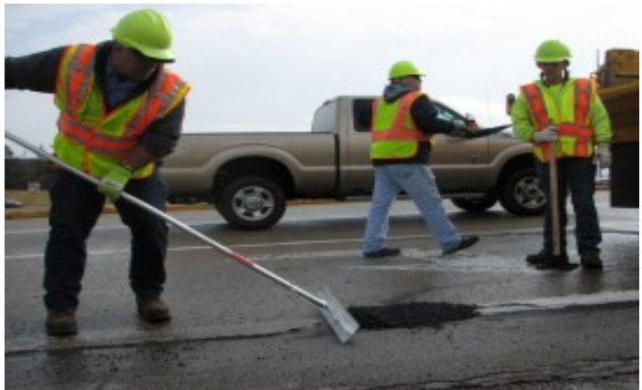
Worker safety, traffic control, equipment, and labor are the most significant costs of repairing potholes.
