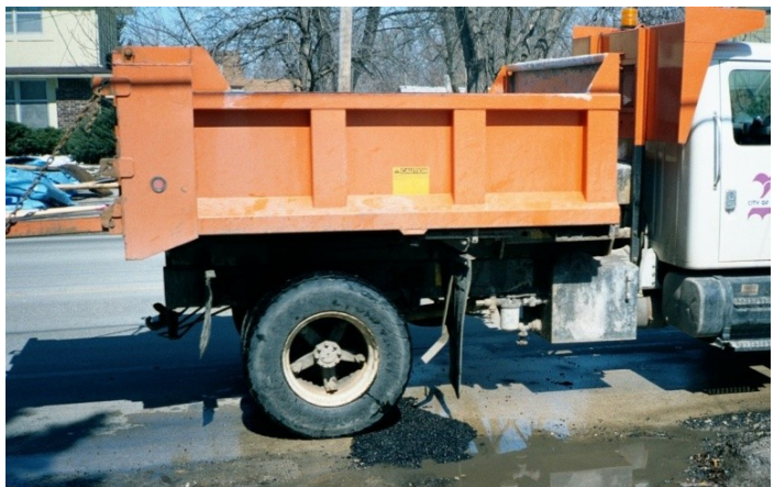
The throw-and-roll method of pothole repairing, in which installed material is compacted by use of the truck, is cost-effective when using a high quality material.
