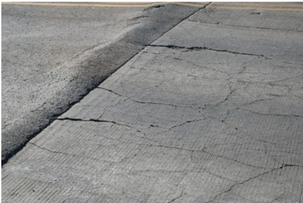
Figure 1 - Several months after construction right in our metropolitan area
