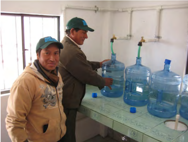
Two of the six system operators trained at the Promisa Divina Church installation in Colta, Ecuador. With the new system up and running, the operators are filling their first bottles of clean water.
