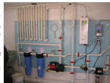
System installation in Colta, Chimborazo, Ecuador (July 2012)
