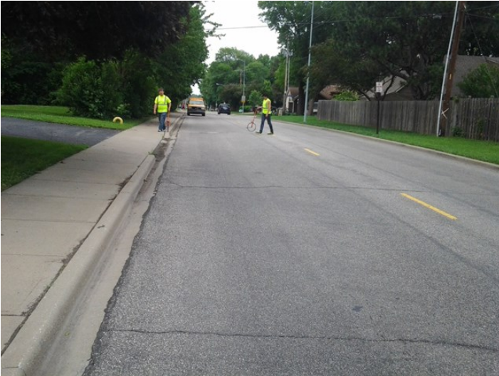
Figure 2 - PCI=54.4 – Lamar near 65 th Street
