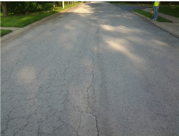
Figure 4 - PCI = 0.0 - Failed condition
