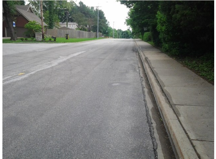
Figure 3 - PCI= 54.4 – Lamar near 65 th Street
